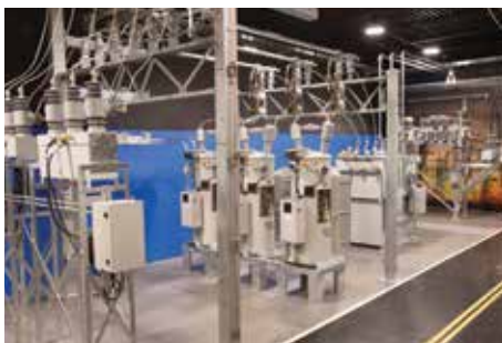
Utility substation and distribution
